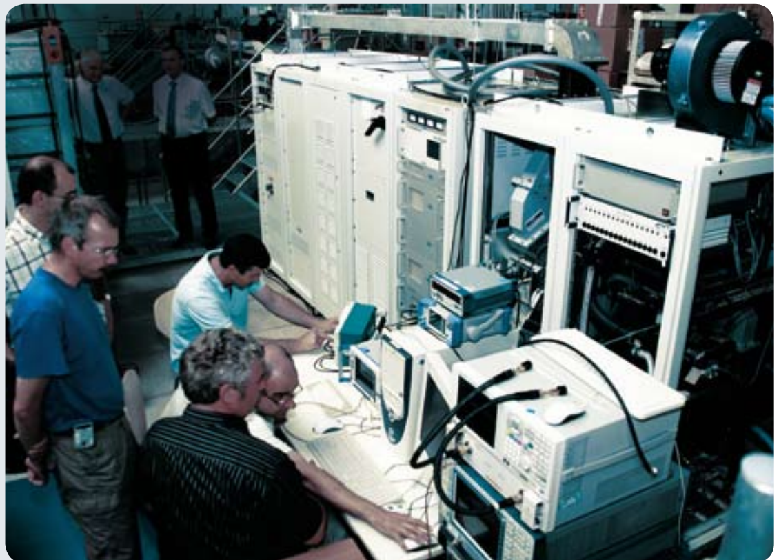
RF IOT high-power transmitter at ELBE FZD Rossendorf, Dresden, Germany.
